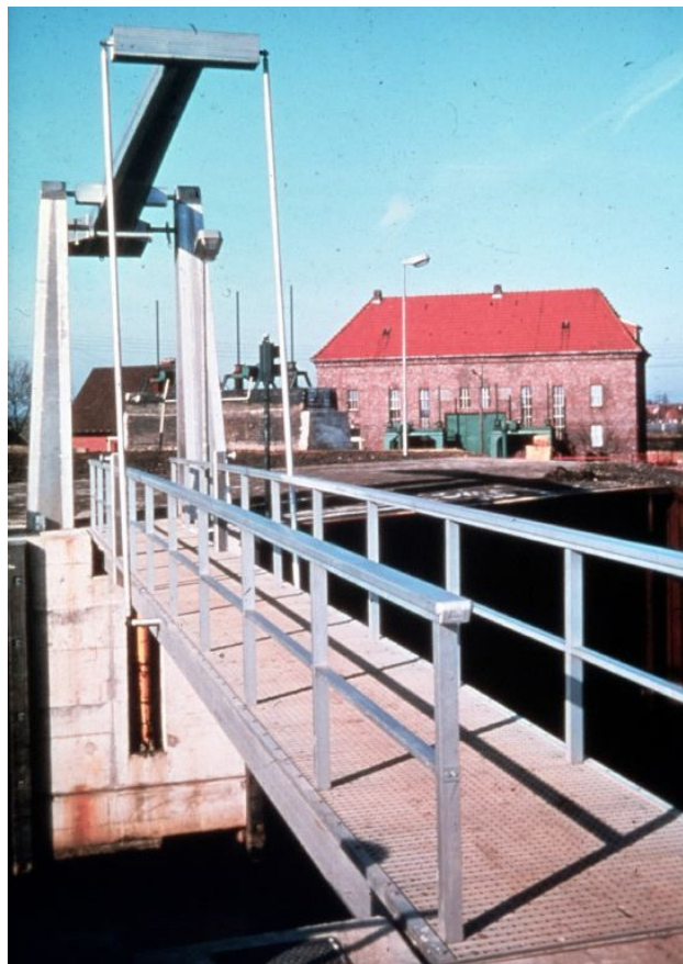
Figure 5: A moving foot-bridge.
